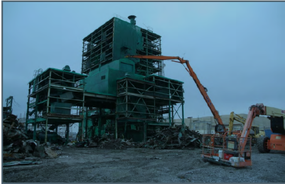
Figure 8-10. Demolition of C-340 building where Uranium and other metals were milled and processed
