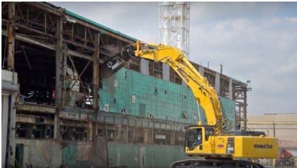
Figure 8-11. Demolition of the C-410 Building where uranium was blended to produce feed material for the enrichment process.
