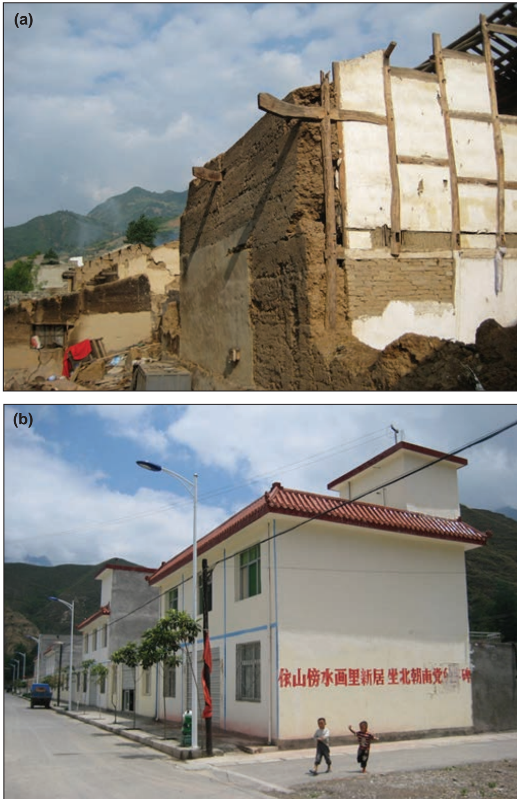
Figure 25. (a) A traditional adobe house and (b) a recently constructed seismic-resistant house after the Wenchuan earthquake. Traditionally built adobe houses suffered severe damage, but houses built to seismic-resistant standards under the government-subsidized mitigation program sustained little or no damage. Photos © Zhenming Wang. Used with permission.
