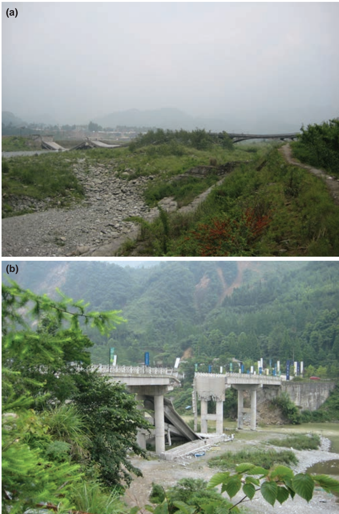
Figure 9. Examples of damage to bridges in the Wenchuan, China, area caused by the May 12, 2008, earthquake. Photo © Zhenming Wang. Used with permission.
