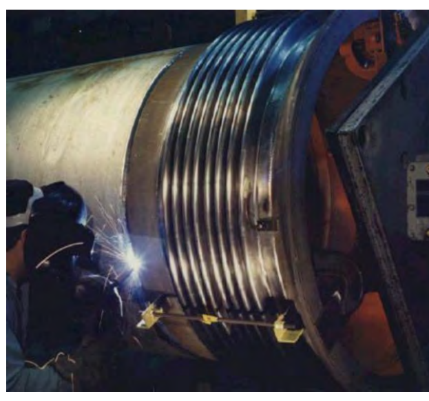
Seismic joints added to Enrichment Process piping in 1998 as part of seismic engineering safety measures.
